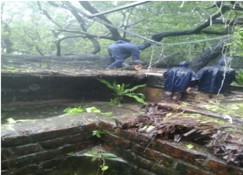
Post-cyclone damage repair
